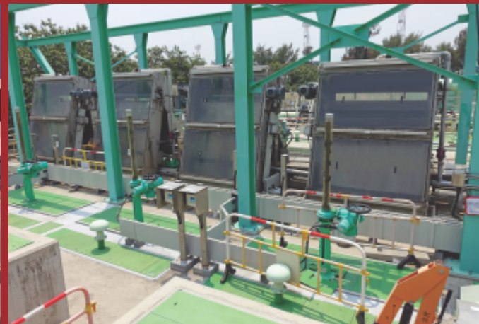
Multirake Bar Screens at Pillar Point STP, Hong Kong
