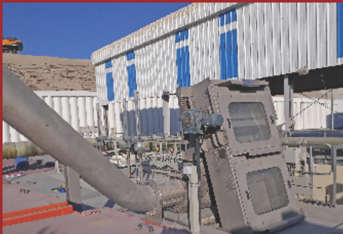
Multirake Bar Screen with Jet breaker installed at Amas STP, Bahrain
