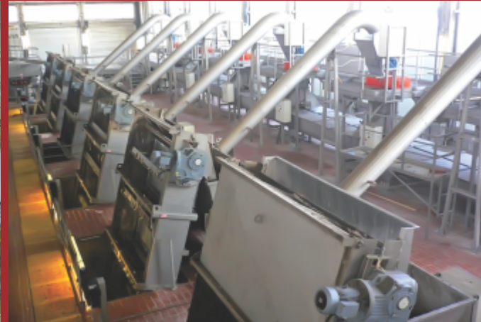
Multirake Bar Screens at Vienna Main STP, Austria
